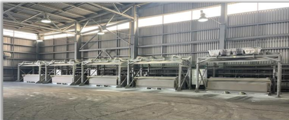
Figure 7. Dross coolers in Ma'aden Aluminium.
